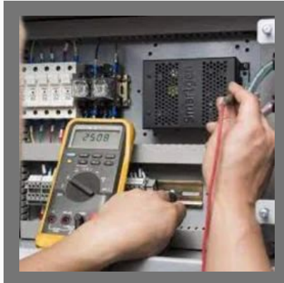
Industrial Online Ups Repairing Services
